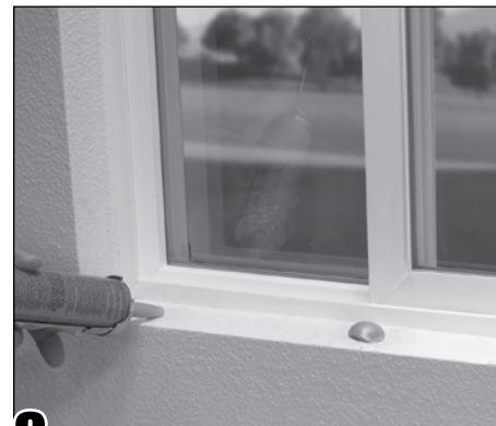
8 Apply 1-inch balls of polyurethane construction adhesive 3 inches from each end and 6 inches on center of the sill area.
