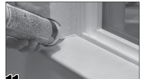
11 Apply a bead of caulk in the joints between the sill and the window, and the sill and the drywall. Smooth the caulk with a wet finger. Occasionally, the butt-cut ends will have voids. These voids can be filled with an all-purpose adhesive caulk.
